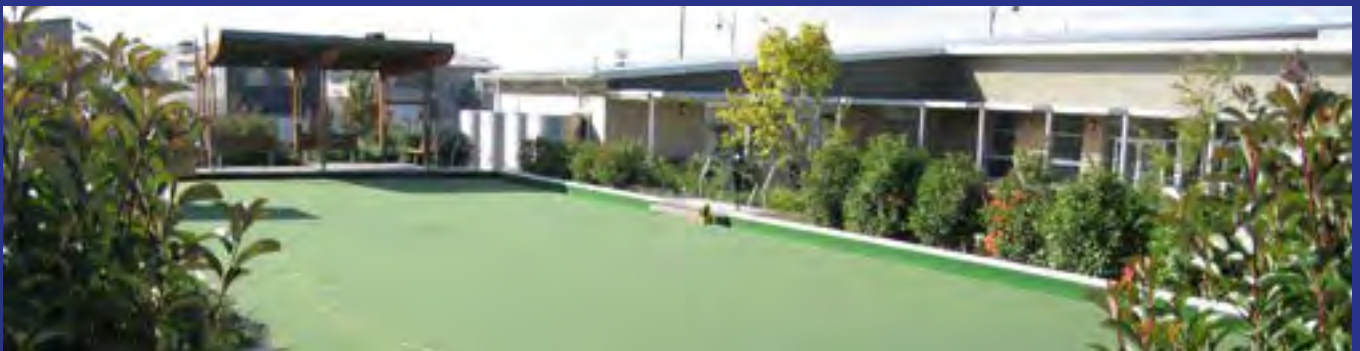
Project: Investigation of Foundation Movement to Bowling Green Services: Forensic Inspections
