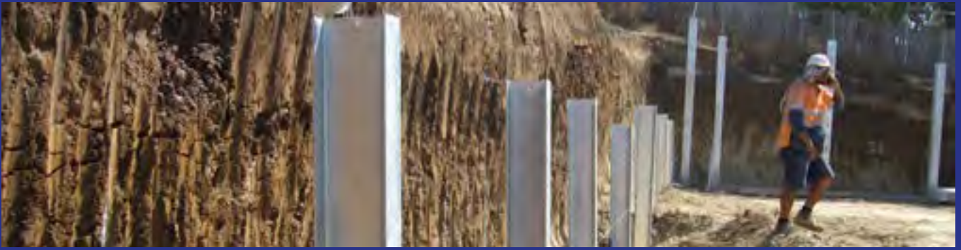
Project: Multi-Unit Residential Development, Westmeadows Services: Structural - retaining wall design Client: Australand Holdings
